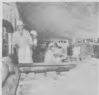
Mechanical Supervisor Dick Bermudez (2nd l) and Donny Henriquez check weatherproofing of insulated fitting under heat exchanger. Applying the mastic (dark) is Mateo Dania. At left, Andres Dijkhoff shows preformed block insulation used. At rear (left) is a completed insulated line with weatherproof mastic partially covered with a gleaming aluminium foil jacket.
